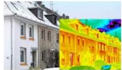
Heat losses observed by thermography
